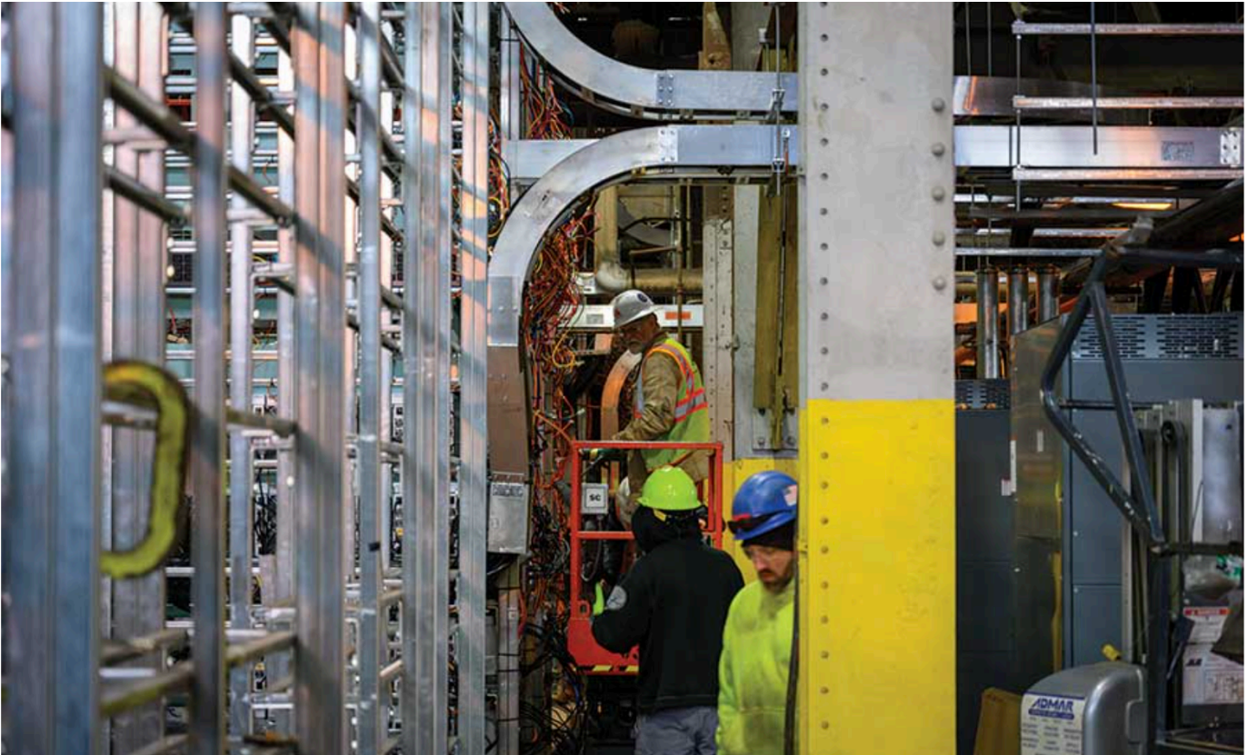
Seven thousand mining rigs were initially to be installed outside the Dresden, N.Y., generating plant, but the noise of the rigs required that they be installed inside the power station.
